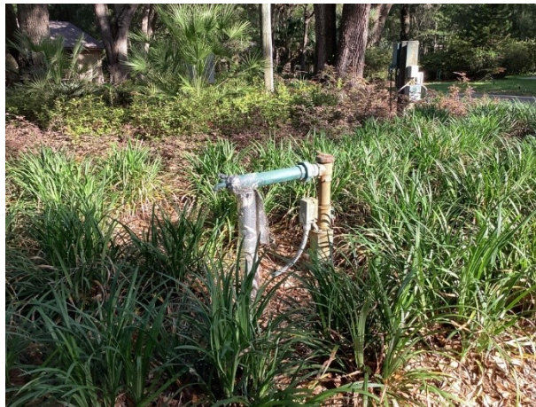
Irrigation equipment at Autumnwood Trail
