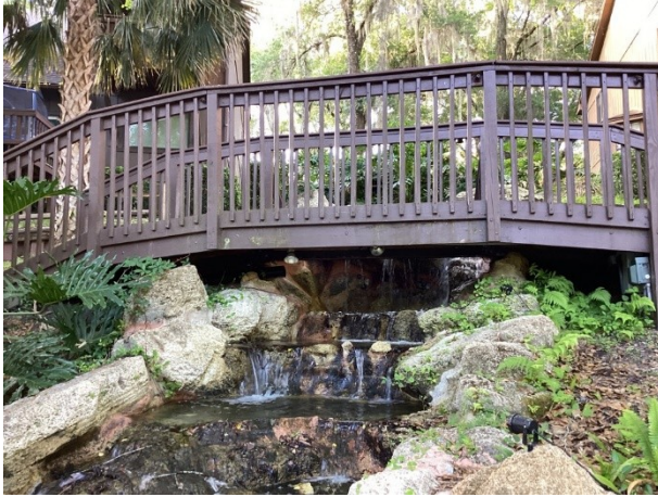
Organic growth at side of bridge
