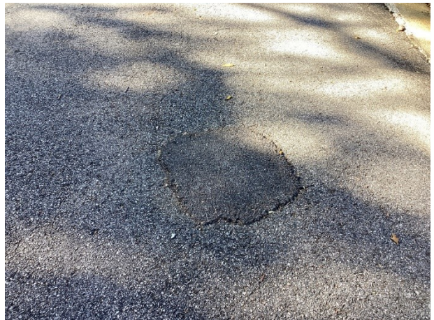
Fill patch at Rosewood Trail
