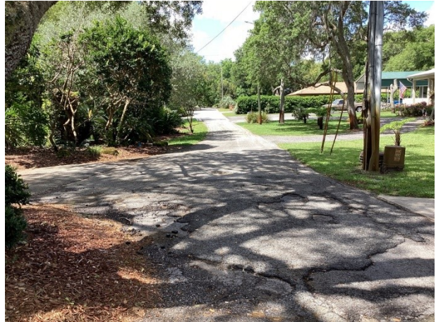
Extensive deterioration at Trail by the Lake
