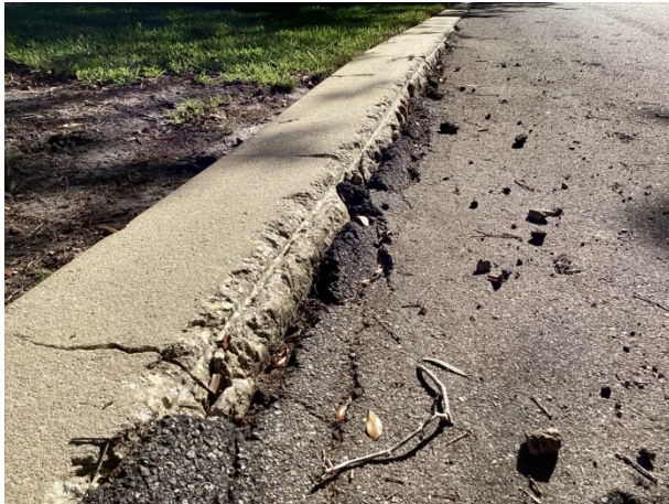
Curb deterioration at Wildwood Trail
