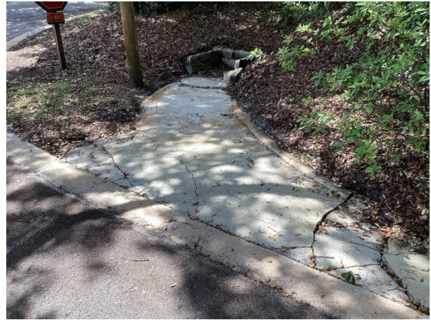
Concrete deterioration leading to catch basin
