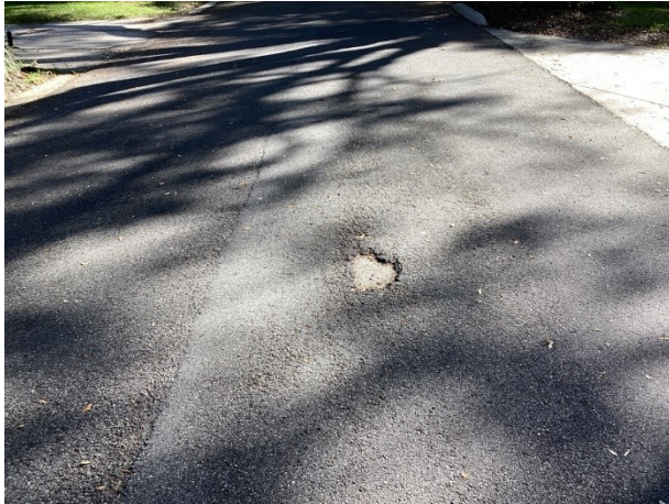
Top layer deterioration at Rollingwood Trail
