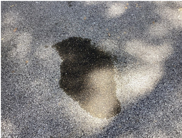
Vehicular stains at clubhouse parking area
