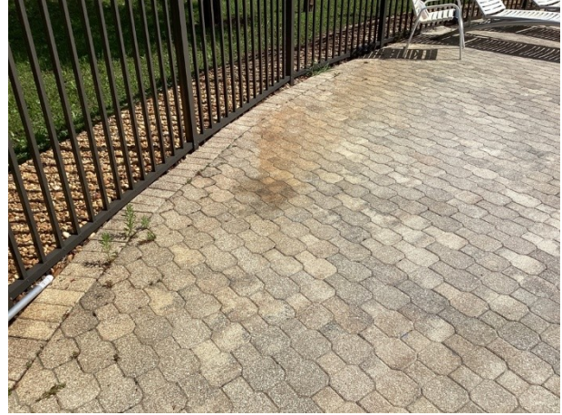
Weathered and stained pavers
