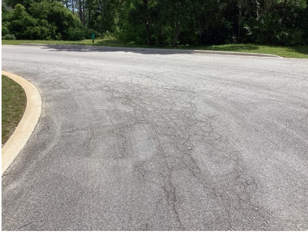
Extensive cracks at Black Willow Trail
