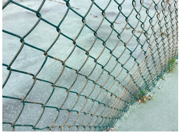
Fence warped webbing with finish deterioration
