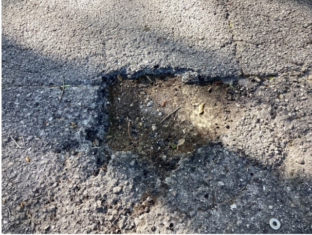
Pothole formation near 810 Shady Branch Trail
