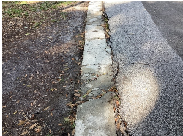
Gutter deterioration along Lone Tree Trail
