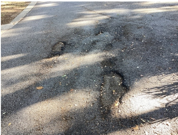
Pothole formation near 10 Autumnwood Trail
