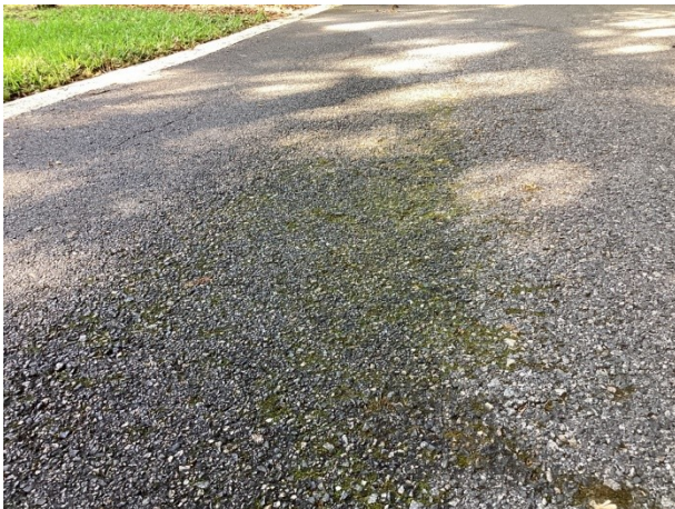
Raveling and organic growth evident along Crooked Tree Trail
