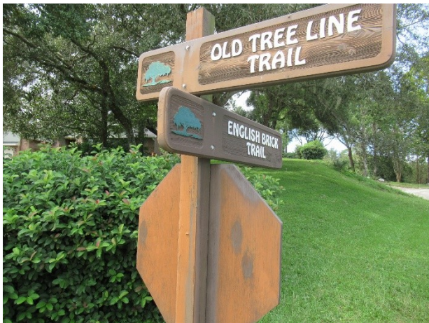
Street and traffic sign with finish deterioration
