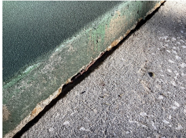
Exposed concrete reinforcement
