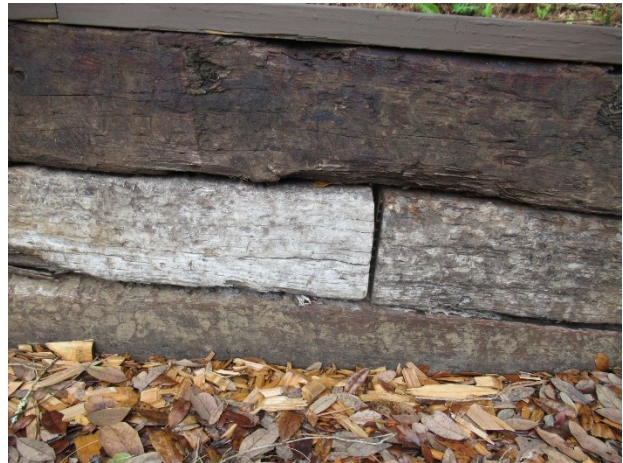
Playground retaining wall with weathered timber
