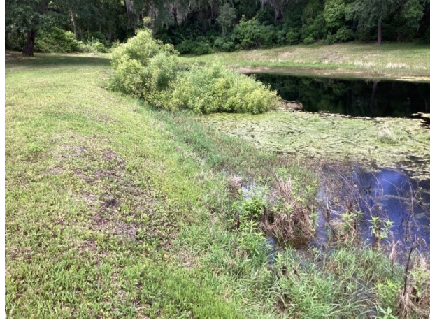
Extensive vegetation at pond north of playground
