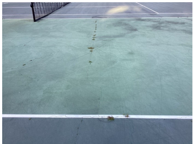
Surface cracks with vegetation
