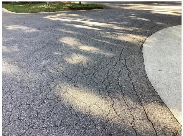
Extensive cracks near clubhouse at Shady Branch Trail
