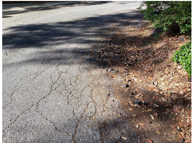
Washout along Black Bear Trail
