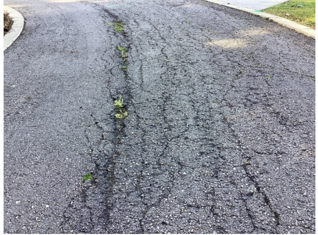
Extensive deterioration near 807 Shady Branch Trail
