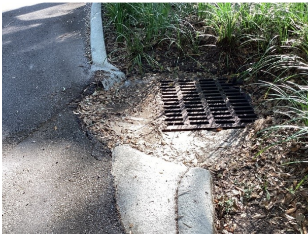
Debris accumulation at catch basin along Woodridge Trail
