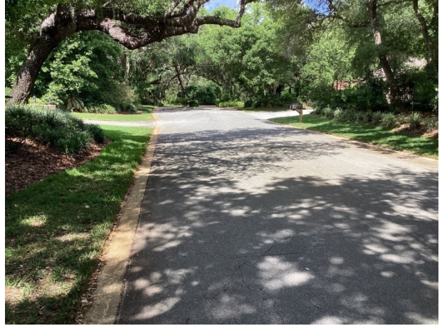
Pavement overview at Black Willow Trail
