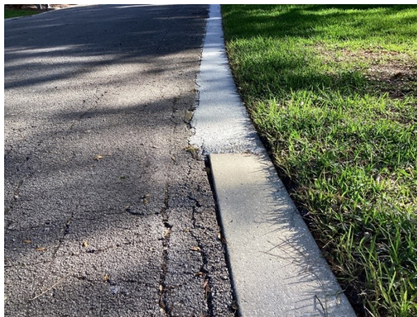
Gutter replacements evident
