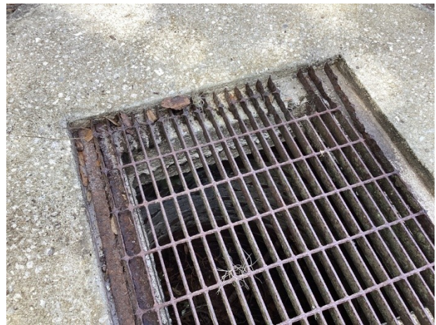
Extensive corrosion at catch basin grate at clubhouse
