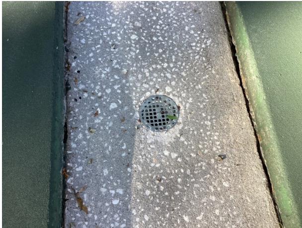
Drainage at shuffleboard court
