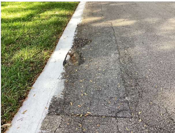
Deterioration at previous patch repairs
