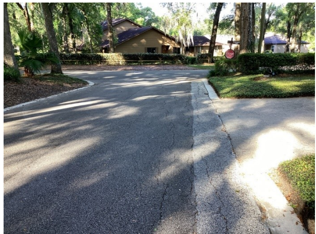
Cracks along Lone Tree Trail
