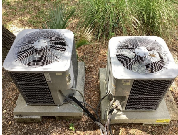
Clubhouse condensing units
