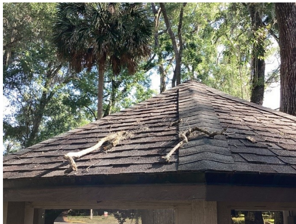
Debris accumulation evident at office roof
