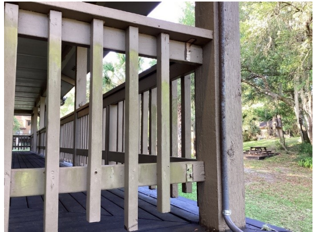
Missing railing picket
