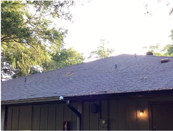
Debris accumulation at clubhouse
