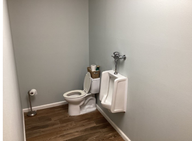
Rest room fixtures
