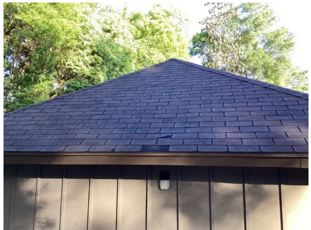
Missing shingles at storage roof
