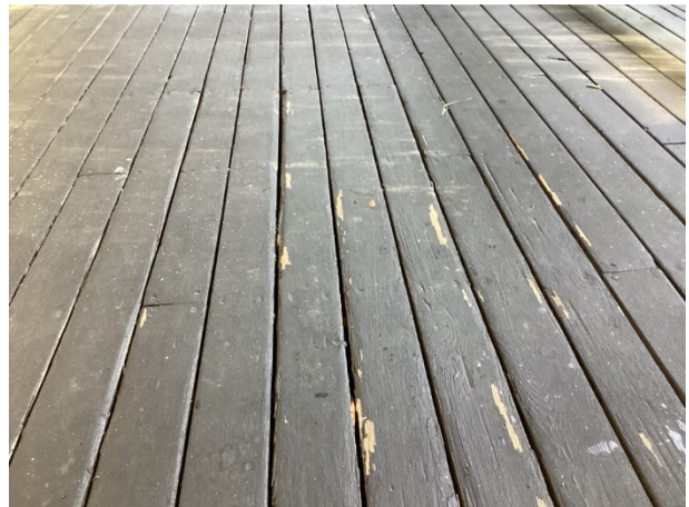
Paint finish deterioration at deck boards
