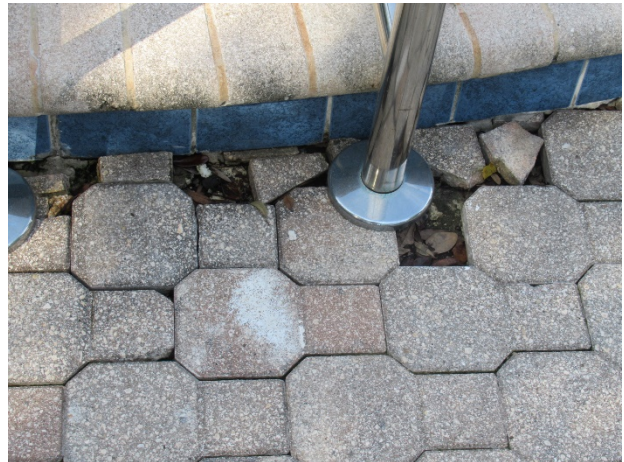
Pool deck with damaged and displaced pavers
