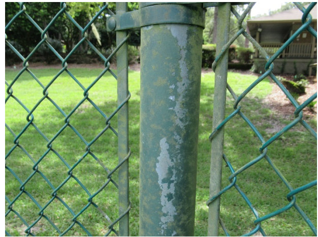
Tennis court fence with stains and finish deterioration
