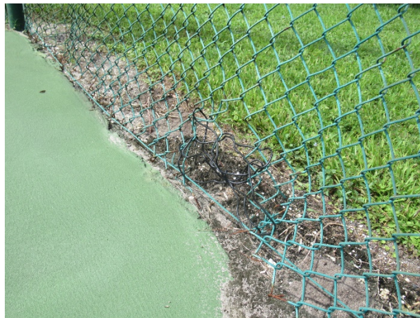
Tennis court fence with past repair evident
