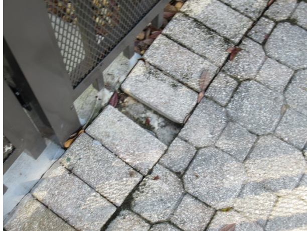
Pool deck with displaced pavers
