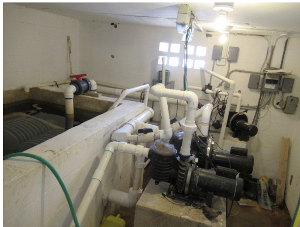
Mechanical equipment overview
