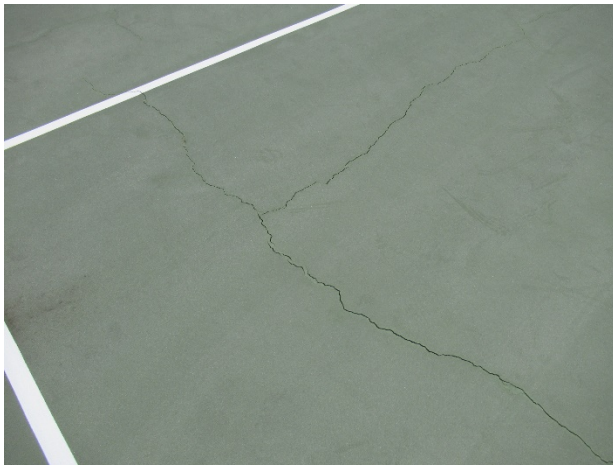
Tennis court surface with cracks
