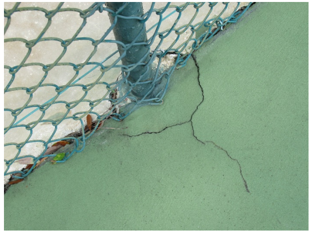
Tennis court surface with cracks around fence post
