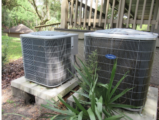
Clubhouse condensing units
