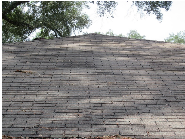
Clubhouse roof overview – note warped shingles
