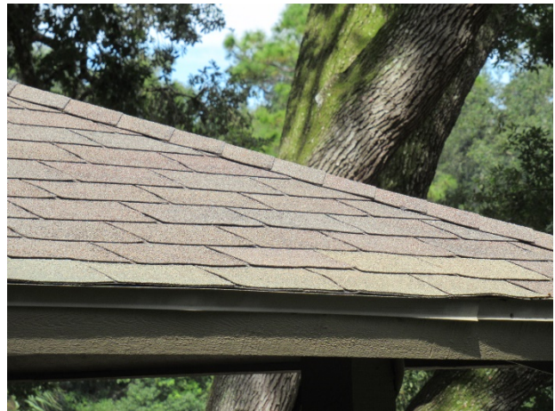
Clubhouse roof with past repair evident
