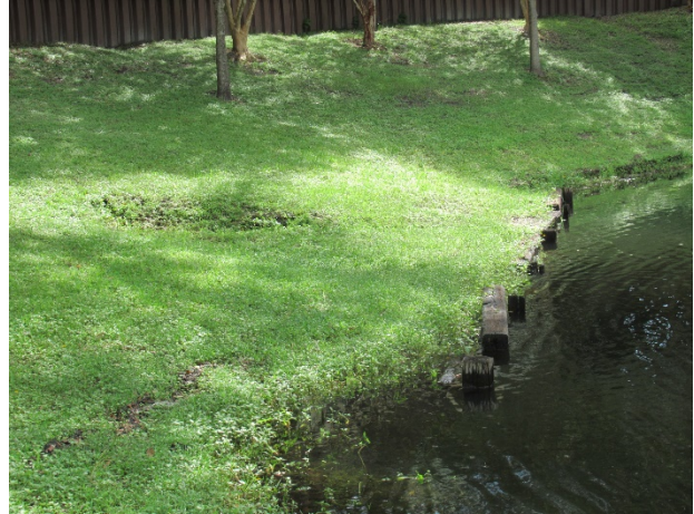
South pond bulkhead – soil erosion is evident in the area behind the wall
