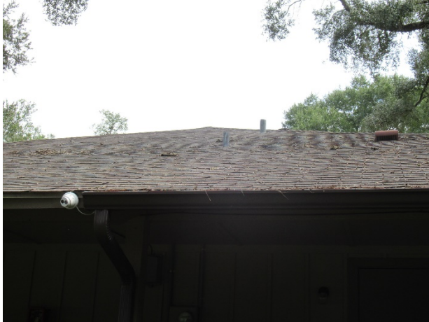
Clubhouse roof with warped shingles
