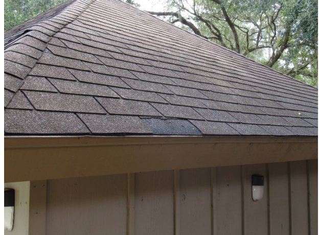
Maintenance shed roof with missing shingle
