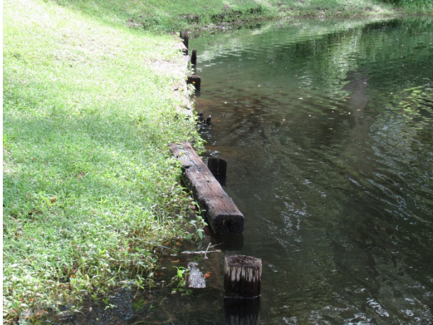
South pond bulkhead – this retaining wall has failed
