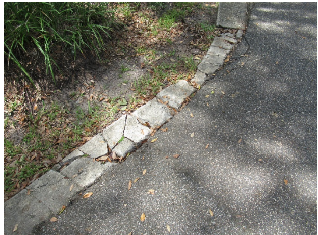
Ribbon curb with severe deterioration – Woodridge Trail
