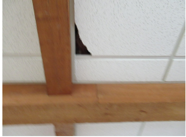
Acoustical ceiling tile with damage
