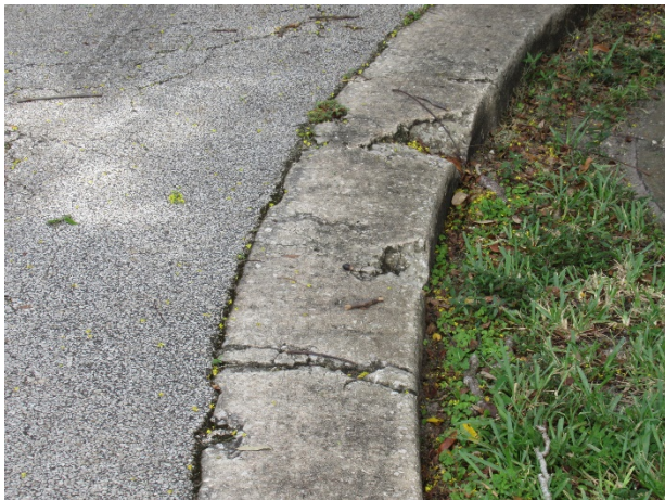
Ribbon curb with cracks – Waters Edge Trail
