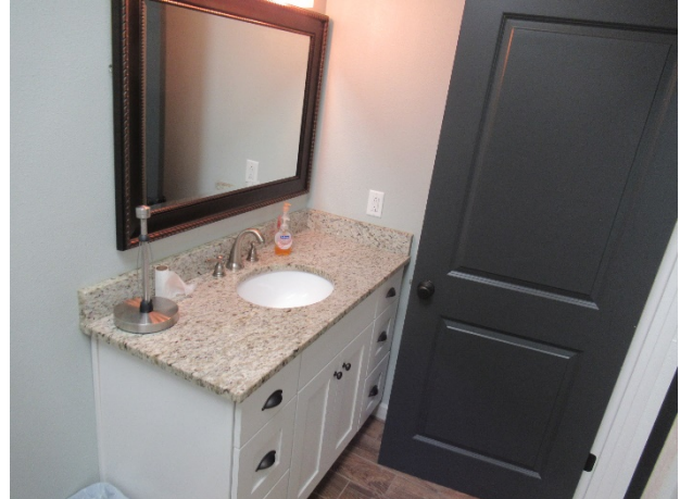
Rest room fixtures
