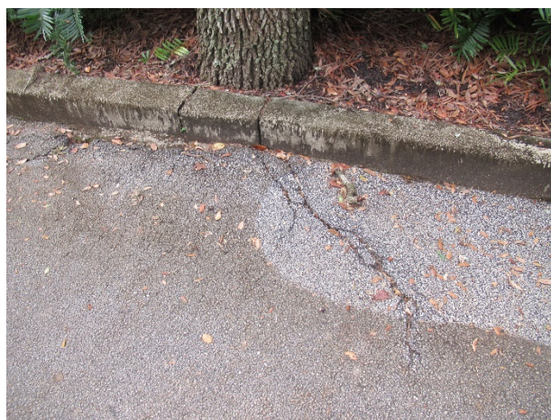
Standard curb with cracks and displacement near tree – Black Willow Trail
