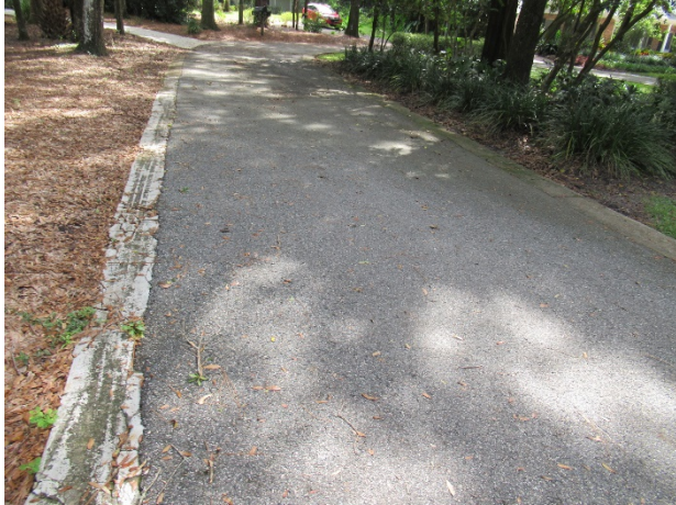
Asphalt Pavement – Circle Oaks Trail
