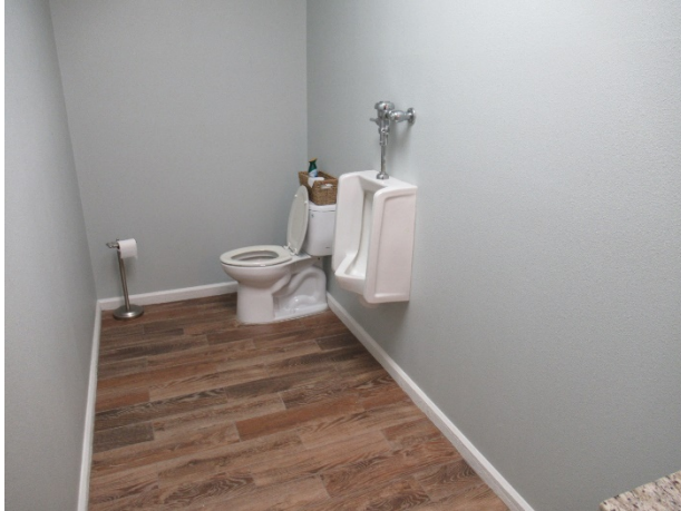
Rest room fixtures
