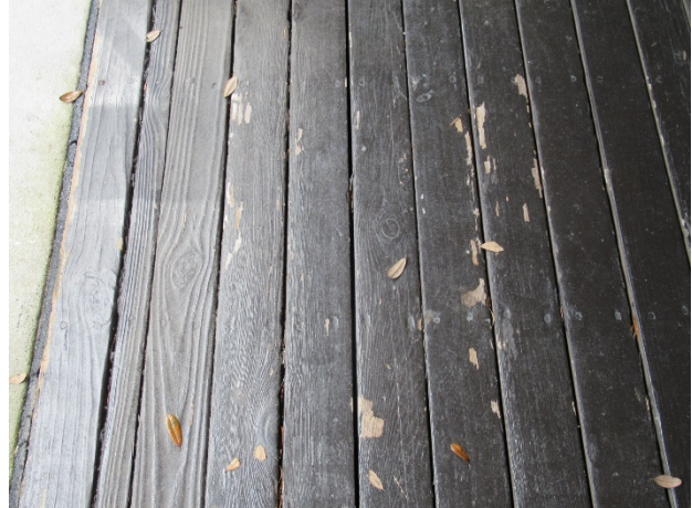
Wood deck with paint finish deterioration
